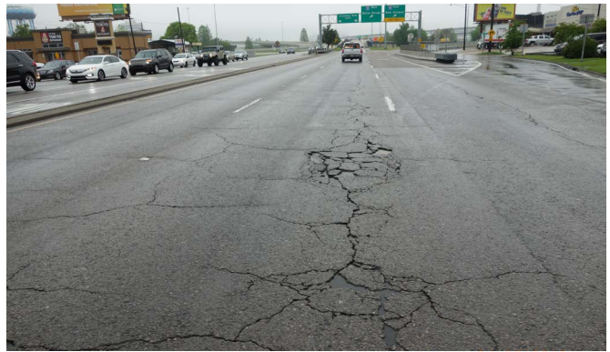
A pavement section rehabilitated without GlasGrid has demonstrated significant cracking over this same time period.
