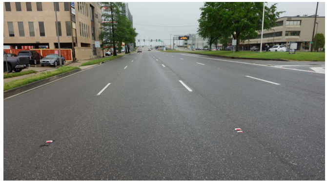
Project site was re-visited in 2019 and very minimal cracking was observed.
