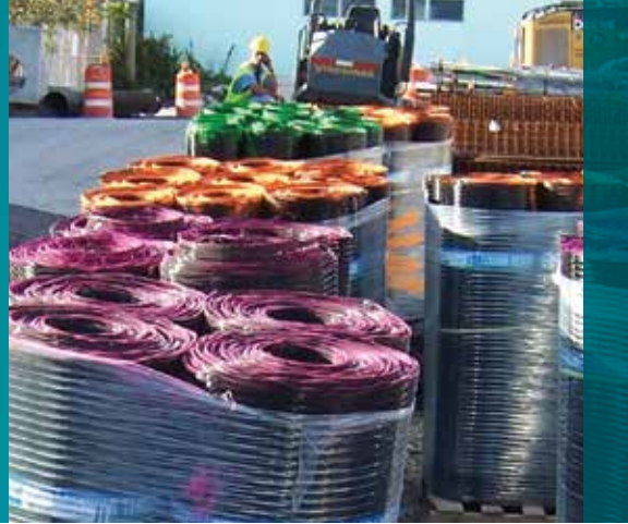
FIGURE 1: Prepare for wall construction by clearing the site and cutting and color-coding the Tensor® Geogrid.
